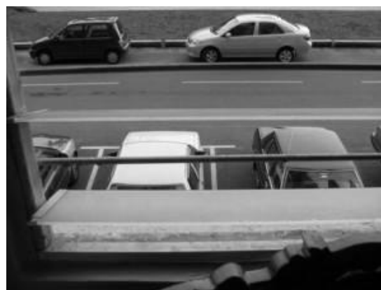
Figure 16: Water splattering due to the coping at the bottom of the window
