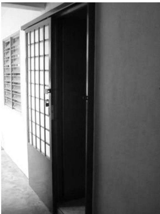
Figure 9: Metal grilles installed at unit entrance door to enhance internal cross ventilation yet not sacrificed safety
