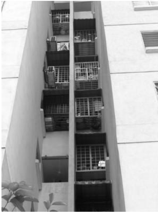
Figure 12: External view of the yard space. The illegal grilles extension at yard space made for cooking and drying purposes. Grilles to prevent thief enter unit via yard space
